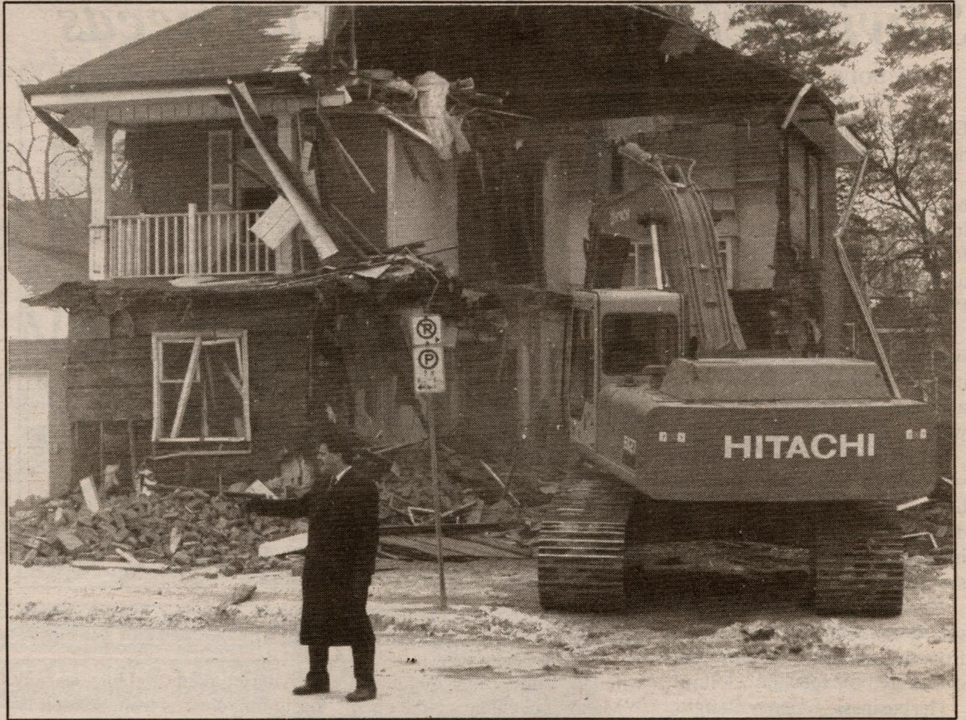
OPEN HOUSE! Captain James Anderson directs traffic as a Mill Street home owned by Acton's Salvation Army is demolished on Friday morning. The lot, which sits directly to the east of the church building, will now be used as a parking lot. If the ground settles properly, the lot could be paved by September. (Steve Martin photo)
