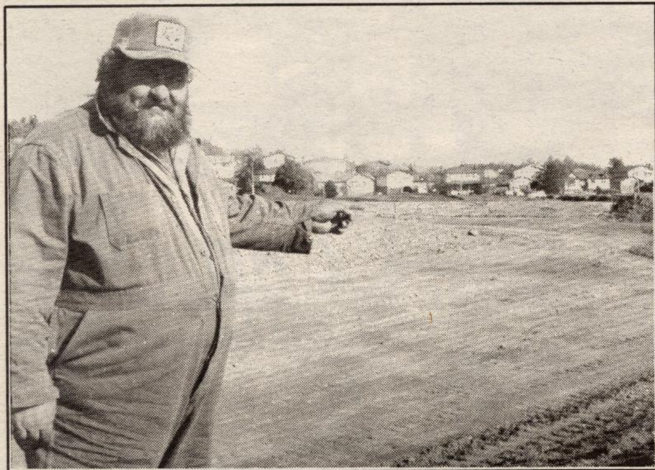
EARLY STAGES: Peter Snow of Nellis Construction points to land beyond St. Joseph's Separate School that will soon house 60 single-family dwellings and a seniors' residence, to be constructed by the Acton Legion. (Doug Harrison photo)
