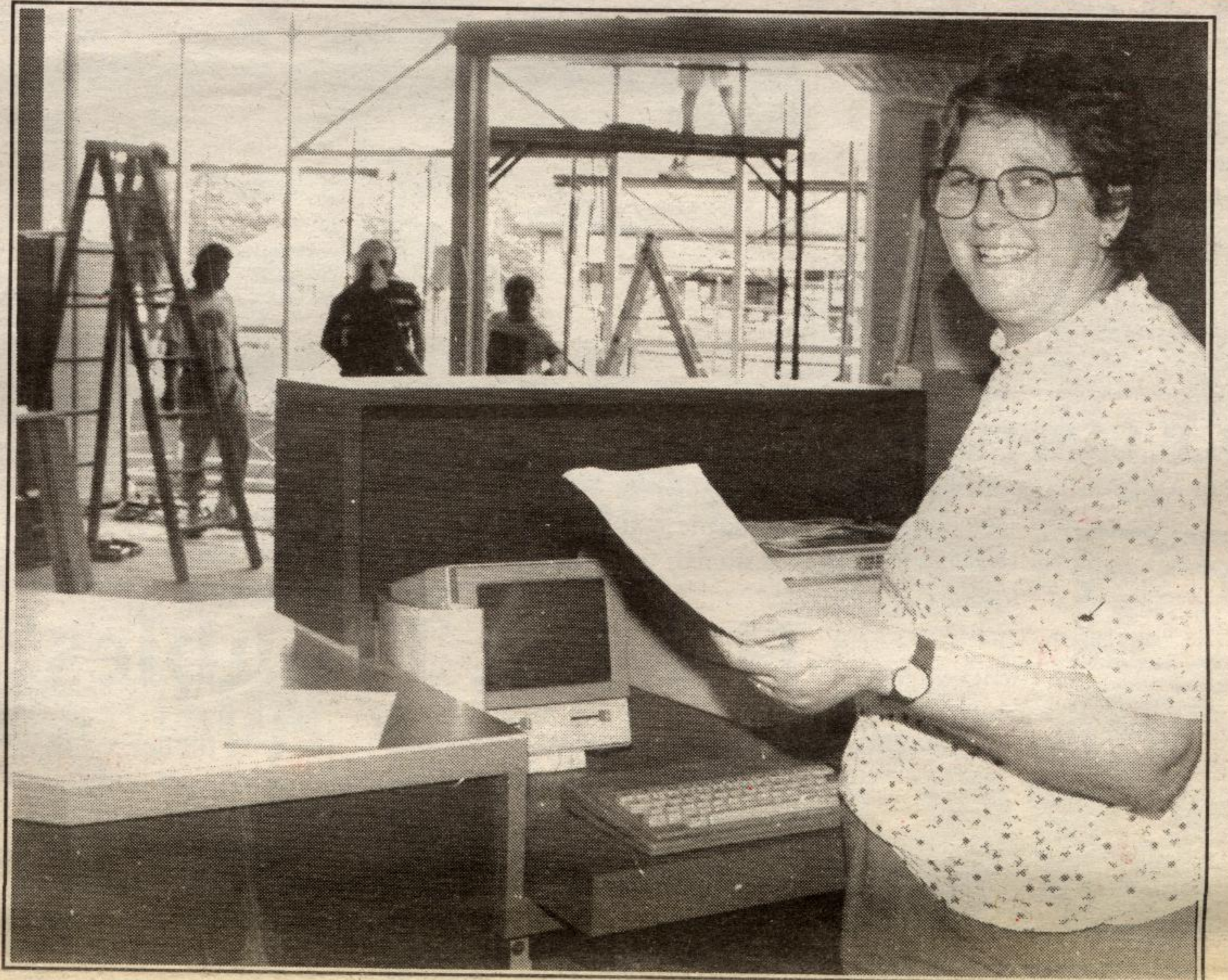
BUSINESS AS USUAL: The Bank of Montreal has kept its front door open for business during renovations even when there was no front door — or front. Last Wednesday even the noise and heat couldn't make Edna Perkons, bank branch manager, lose her smile. (Tim Morgetroyd photo)
