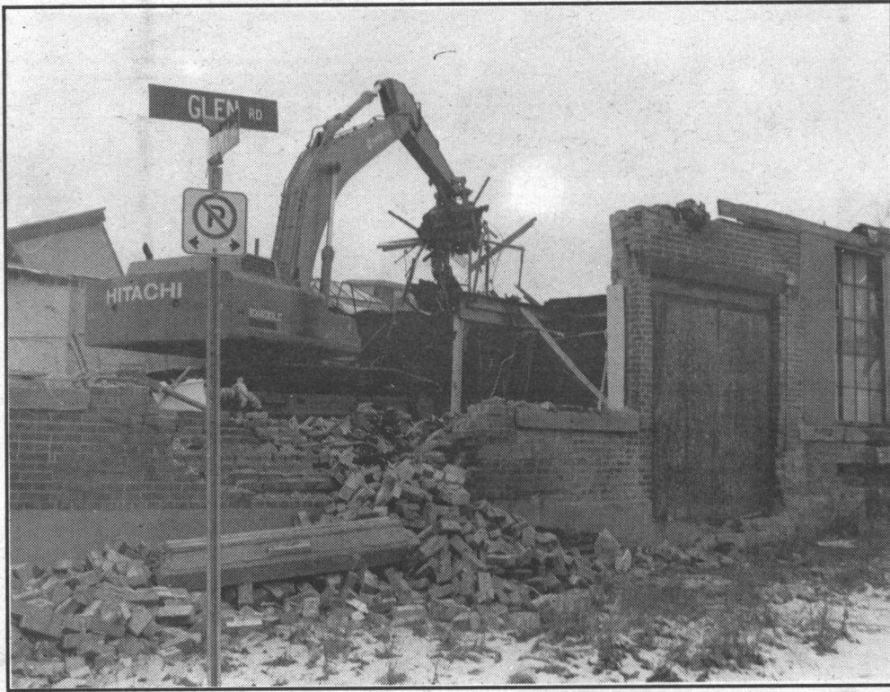
The old Smith and Stone building on Glen Rd. in Georgetown, an industrial landmark for almost 70 years, was demolished in mid-December after being closed for more than a year. photo by Oksana Buhel/HHTW
