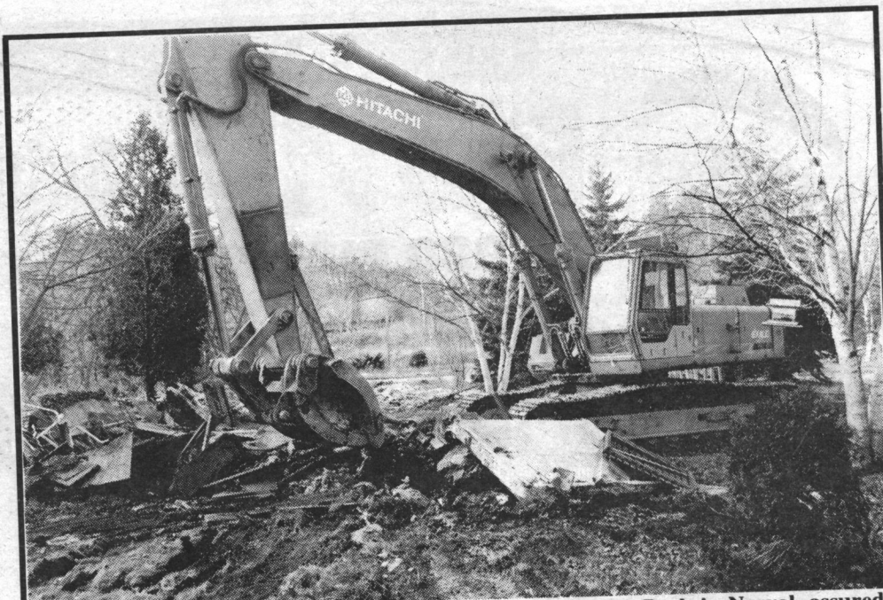
Health and safety issues are no longer a concern at Willow Park in Norval, assured Ken Owen, manager of the Credit Valley Conservation Authority (CVCA), which owns the property. The work was completed Thursday by Cardinal Waste Management of Etobicoke, at a cost of $9,000. The project was tendered Oct. 1, but Owen explained faulty equipment prevented the clean-up from starting on schedule. photo by Simon Wilson/HHTW
