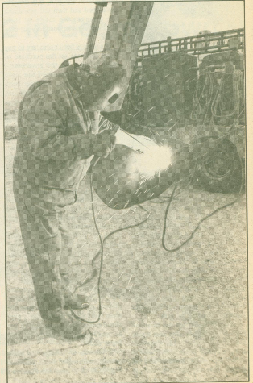
Welder Roy Hickson, with Rowad contracting, takes some time out for quick repairs to the backhoe scoop, during a Consumers Gas project on Highway 7, as the crew installs a gas line to the Jehovah Witness meeting hall. Consumers Gas pipeline inspector, Scott Osborne, said the project is slightly behind schedule because of foul weather, but should be completed soon. Photo by Laura Salverda
