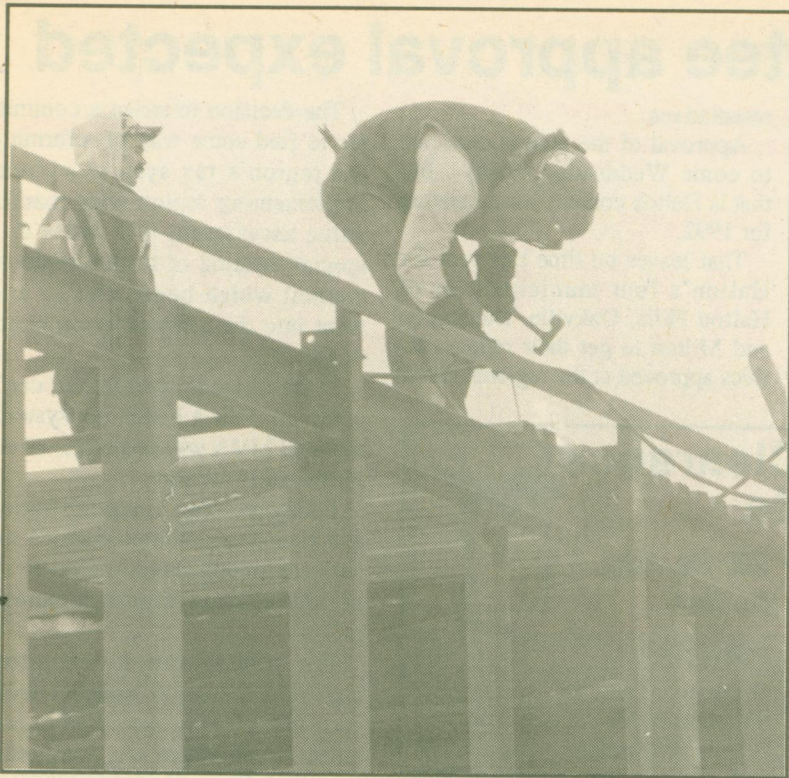
Despite blustery winter conditions these construction workers continued work on renovations of the Georgetown Canadian Tire store. The work is expected to continue through the winter.
