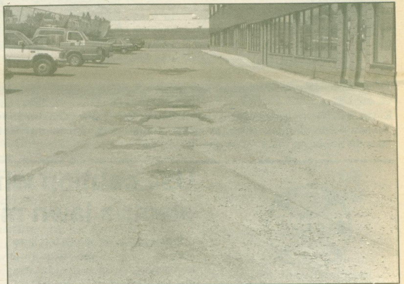
Williams' Armstrong Ave. condo unit requires repairs to its parking lot and other areas.
