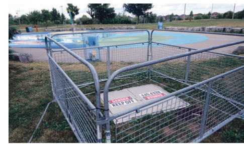
The Town of Halton Hills erected a fence around the metal doors to the Gellert Centre's splash pad control box after a Brampton boy burnt his feet severely one hot summer day.
