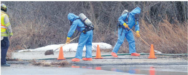
Firefighters shovel dirt around a grate to prevent sulphuric acid leaking from a tank car at the top of a hill into the sewer system. Photo by Eamonn Maher
