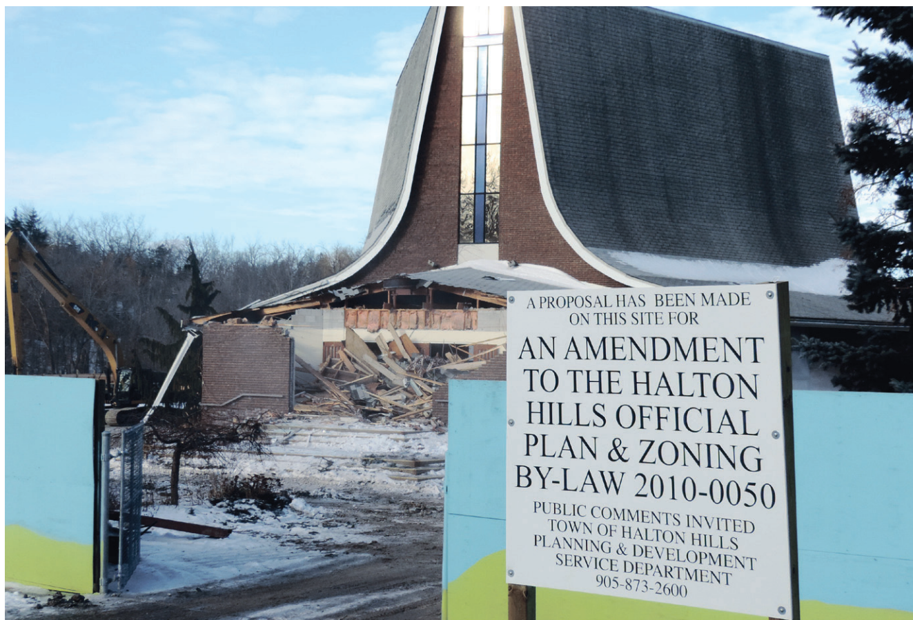
DEMOLITION BEGINS: Demolition of the former Holy Cross church on Maple Ave. is under way to make way for a proposed 120-unit retirement residence. Rockport Group has filed an application with the Town seeking Official Plan and zoning bylaw amendments to allow for the six-storey building. A public meeting on the application is set for Monday (Jan. 26) 6:30 p.m. in the Council Chambers.
