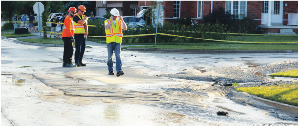
Halton Region crews worked through the night to fix a water main break last Friday. Photo by Alex Docker
