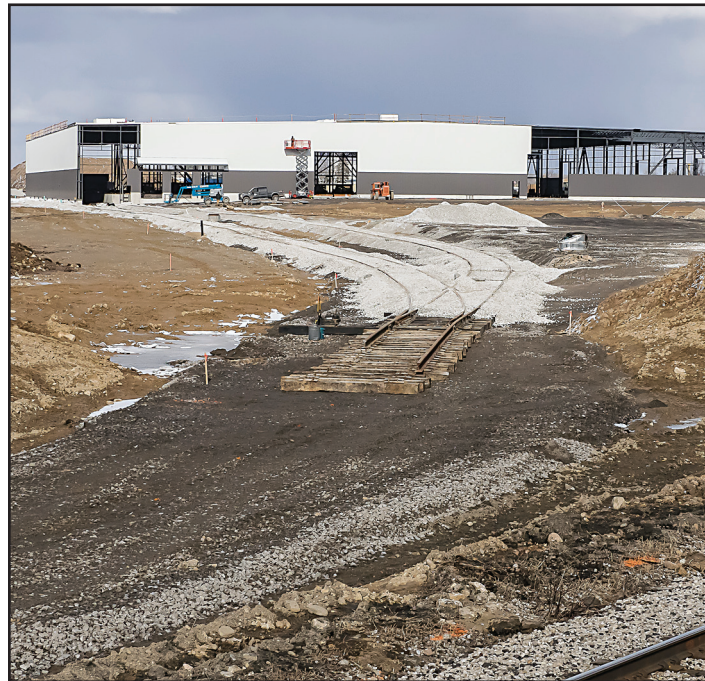
QUICK WORK: A relatively easy winter has allowed for steady progress at the new industrial park in Acton. In this photo taken last week, metal siding was starting to go up on the building, and crews were getting ready to connect the rail spur to the main line. By Tuesday, the metal siding installation was nearly complete and the rail spur connection had been made. - Les Schmidt photo
