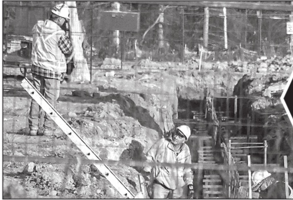
BREAKING GROUND: Purity Life has broken ground on a 30,000 square foot expansion of its facilities on Commerce Court in Acton. They expect to have the work completed in the fall 2017. - Les Schmidt photo
