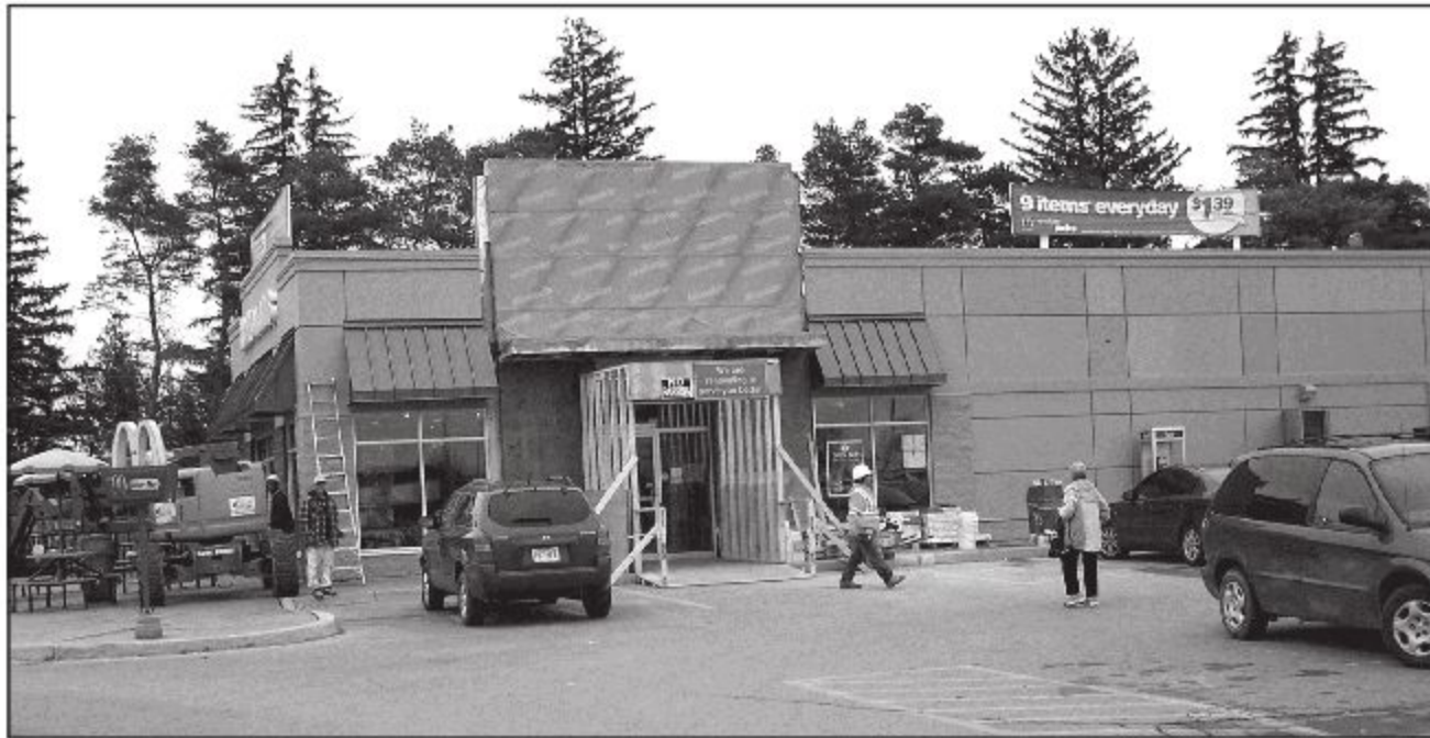
ARCH APPEAL: The interior refurbishment at the Acton McDonald's should be wrapped up next week, and the major exterior work – a brand new corporate look – is also almost complete. – Marie Shadbolt photo
