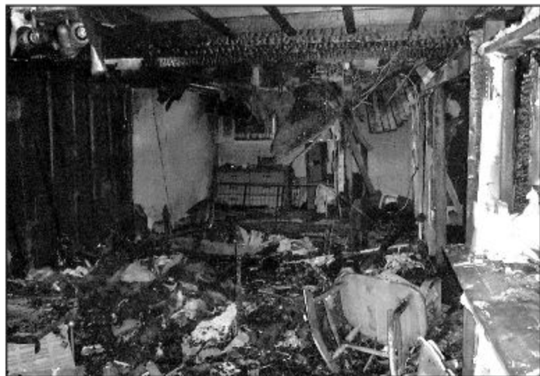
FLAMING INFERNO: The aftermath of this raging fire, sparked by a marijuana grow op in an illegal basement apartment in Georgetown, was fuelled by improper construction, no fire separations and under-rated fire doors. In response, the Fire Department initiated a Home Safe Home free fire safety inspection pilot program which will run for Fire Prevention Week from October 9 to 15. – Submitted photo
