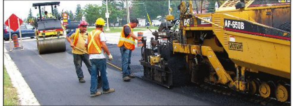
CONSTRUCTION COMPLETE, FINALLY: Many Acton motorists are very happy that the $993,000 reconstruction of Wallace Street (top) is complete, and the road, with a new three-metre wide bike/walking path, is open. Some of those drivers also breathed a sigh of relief when crews finished repaving Queen Street late last week. – Ted Tyler/Frances Niblock photos
