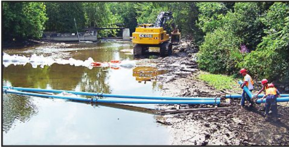
RIVER CROSSING: Crews lay temporary water lines across the Eramosa River in Rockwood last week in preparation for installation of new pipes under the bridge. – Marie Shadbolt photo
