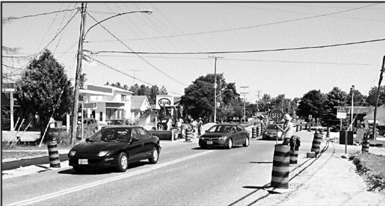
EXPECT DELAYS: The $7-million reconstruction of Highway 7 in Rockwood means delays for motorists, but one lane of traffic will be open at all times while crews install new curbs, sidewalks and repave the highway from the Rockwood Conservation Area to George Street. Next year, the remainder of High-
