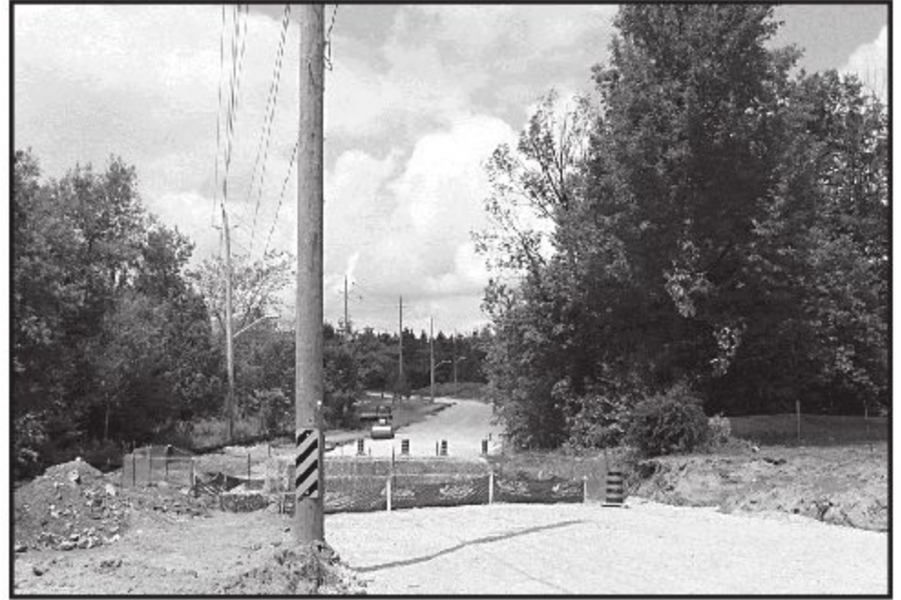
AHEAD OF SCHEDULE: The reconstruction of Wallace Street from McDonald Boulevard to Dr. Moore Court is on budget and ahead of schedule. The work will be complete by mid-to-late September. - Frances Niblock photo
