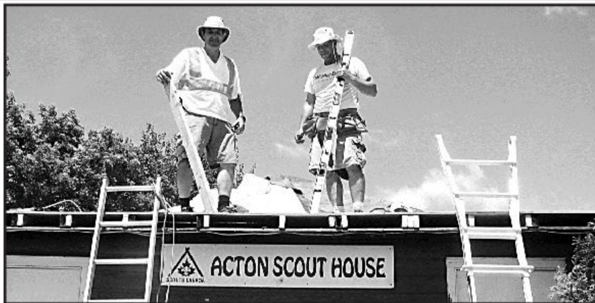
BE PREPARED: With building supplies purchased with donations from the Acton Legion and other donors, Scouter George Henderson (left) and Conall Doherty worked on putting a new roof on the Scout House. – Submitted photo
