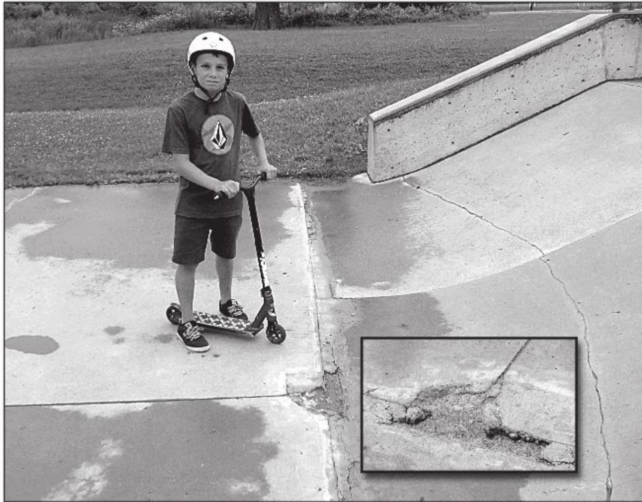
CRACK CONCERNS: Users of the Acton skateboard park, including Acton's Eric Mackenzie, 12, know to avoid the many patched cracks and holes at the seven-year-old facility at the Acton arena/ community centre. – Frances Learment photo
