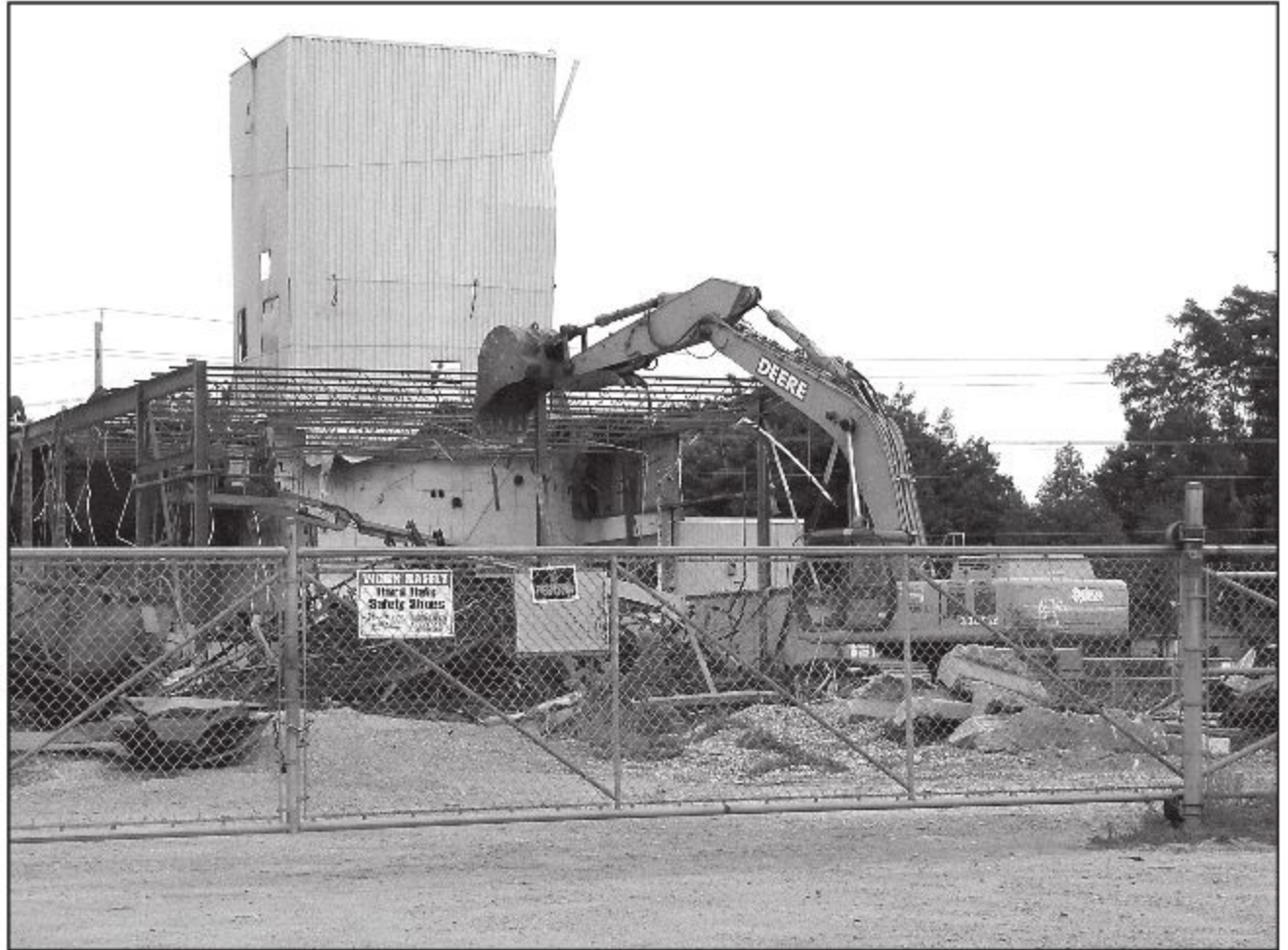
DEMO UNDERWAY: By the end of next month, the former Holly Industries plant on Eastern Avenue will be levelled. The sulphur manufacturing plant was closed by its American owners following an explosion and fire at the plant last November. – Frances Learment photo
