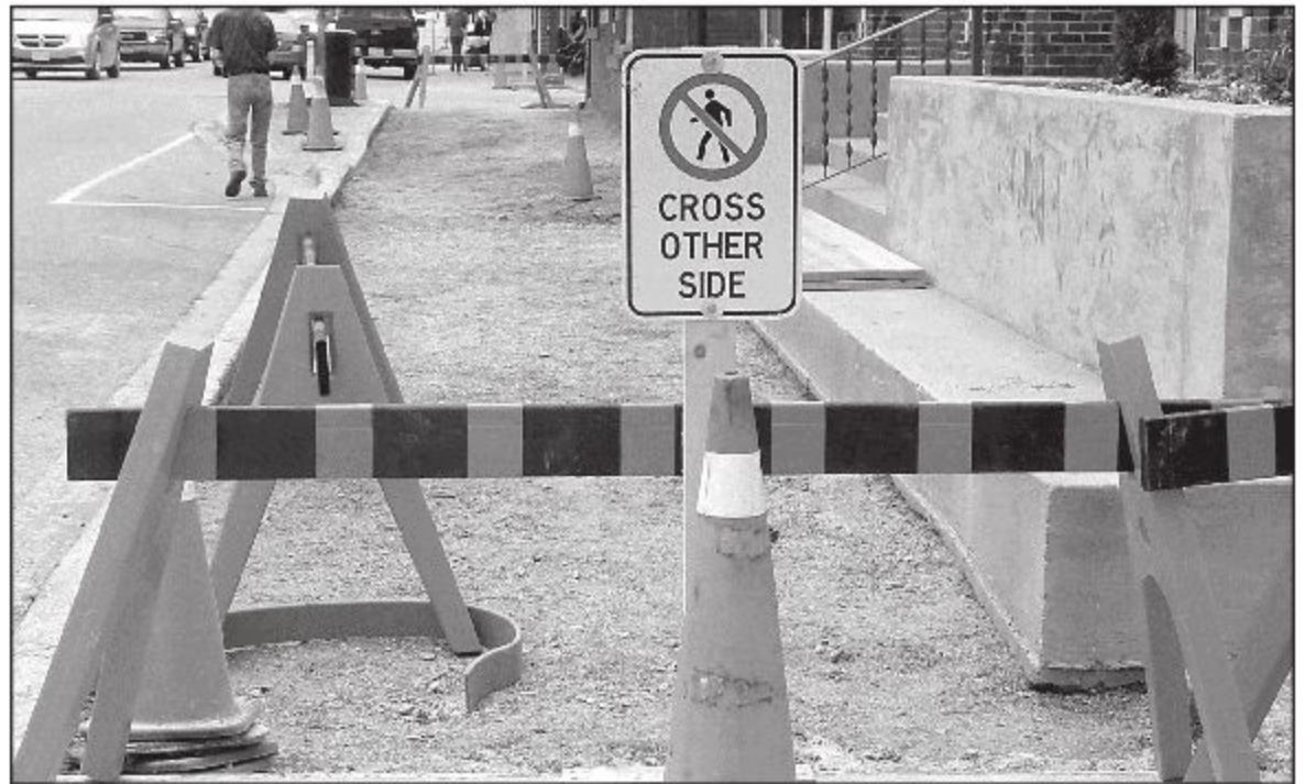
SIDEWALK REPLACEMENT: Town works crews hope to finish replacing the sidewalk on the north side of Mill Street between John and Willow Streets this week, after completing the south side last week. If there is any of the $25,000 budget left, crews will continue heading easterly, removing the crumbing and uneven interlocking brick and replacing it with longer-lasting concrete. – Frances Learment photo
