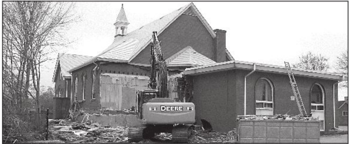
ACCESSIBLE KNOX: The old choir room was demolished at Knox Presbyterian Church to make for an extension which will house an elevator, a new choir room, storage and meeting space, along with a new back entrance. Construction should be complete by the end of the summer. – George Henderson photo
