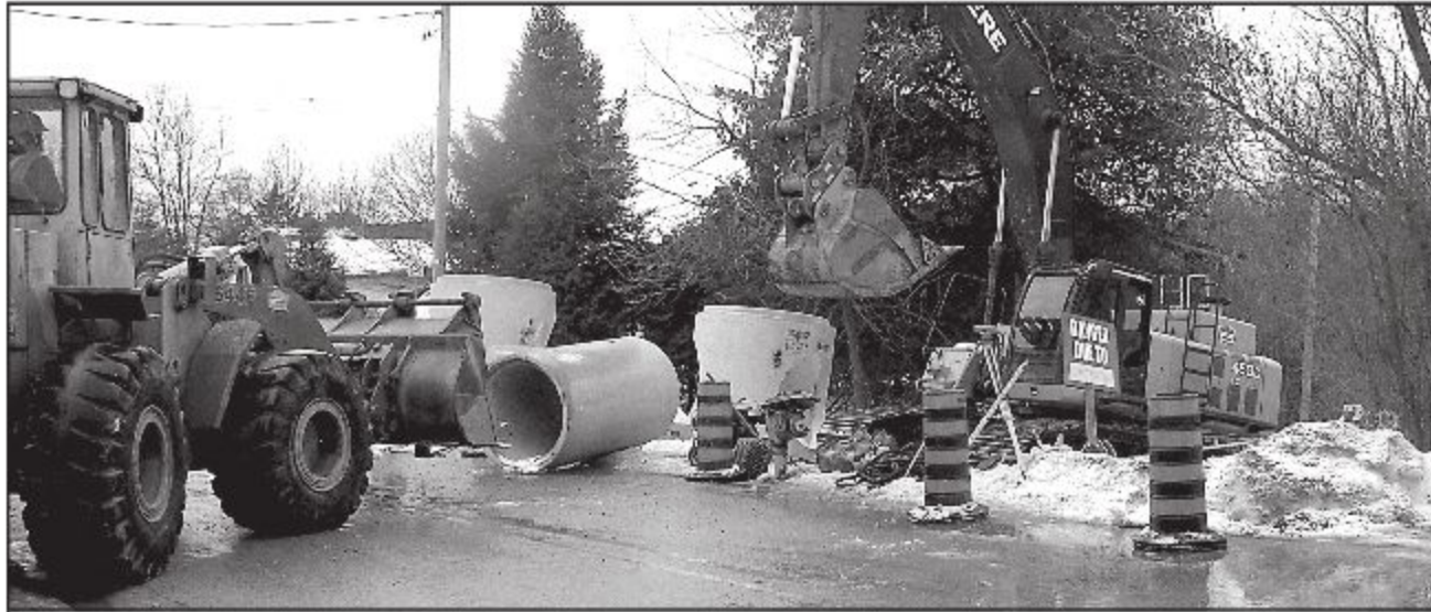
CONSTRUCTION CLOSURES: Harris Street will be closed intermittently over the coming weeks as crews install a huge drainage pipe designed to prevent any further flooding due to the Noble Ridge housing construction. Last month, a torrent of mud and debris flooded Harris Street when two subdivision storm water management ponds failed. — Marie Shadbolt photo
