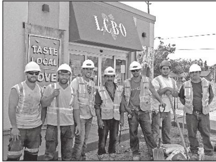
PAVING PARADISE: Jamie Jacome, Jason Inacio, Brian Coelho, George Moura, Andrew Correia, Michael DaCosta, and Sergio Coelho have been working hard this past week enlarging and resurfacing the LCBO parking lot and putting in a new sidewalk. There are future plans to remodel the inside as well, although the details of when and how much have not yet been finalized. – Kate Hendry photo
