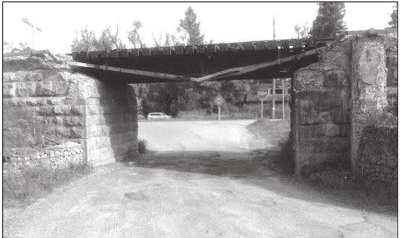
BUNGEE CORD REPAIRS: A Crewson Corner resident is unhappy with the repairs done to this rail underpass off Highway 7 at the junction of Halton, Erin, Eramosa and Milton. - Submitted photo
