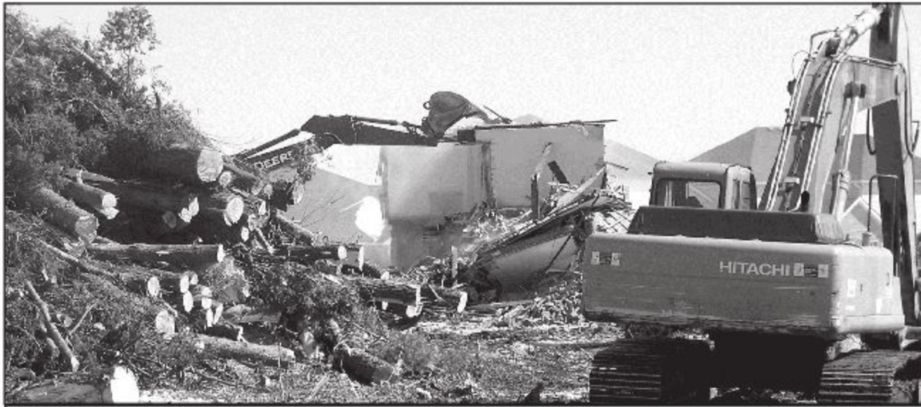
SITE PREPARATION: On Friday, crews continued to clear the future Acton home of a No Frills food store on Queen Street. Shoppers could be in the aisles by October. - Marie Shadbolt photo
