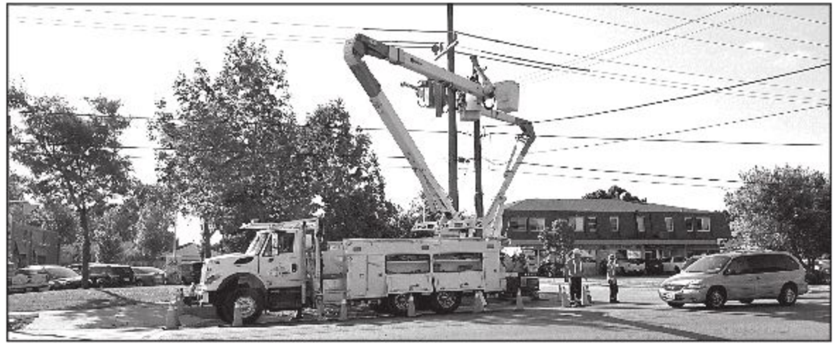
HYDRO TEAMWORK: Crews were busy on Tuesday morning at the corner of Hwy 7 and Meadvale Road performing maintenance at the top of the Hydro poles. - Iain Brennan photo
