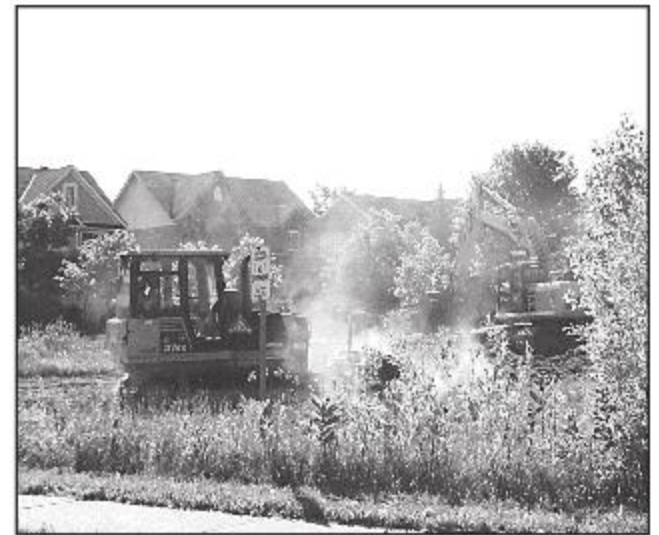
BREAKING GROUND: Workers break ground at the Noble Ridge plaza site Tuesday morning. The site will be cleared to make way for several retail businesses in two buildings. - Vivien Fleisher photos
