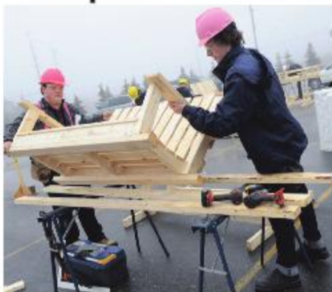
Georgetown District High students Timothy Wingfield (left) and Josh Wiensczyk work on their wooden bench project during last year's skills competition.
