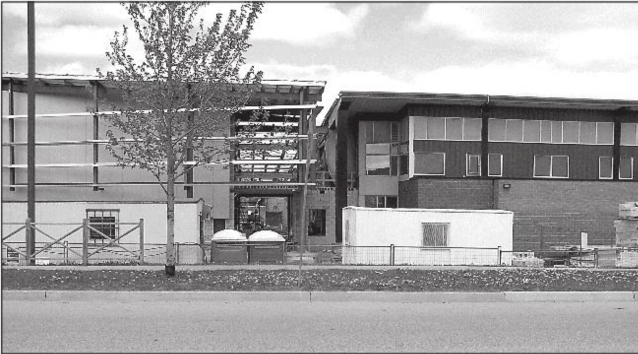
ARENA PROGRESS: Work continues on the expansion of Acton's Arena. - Marie Shadbolt photo
