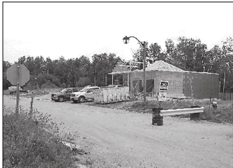
HERE WE GROW: Work has begun on the Trinity Court development in north Acton. The nine home project is partially sold. - Iain Brennan photo
