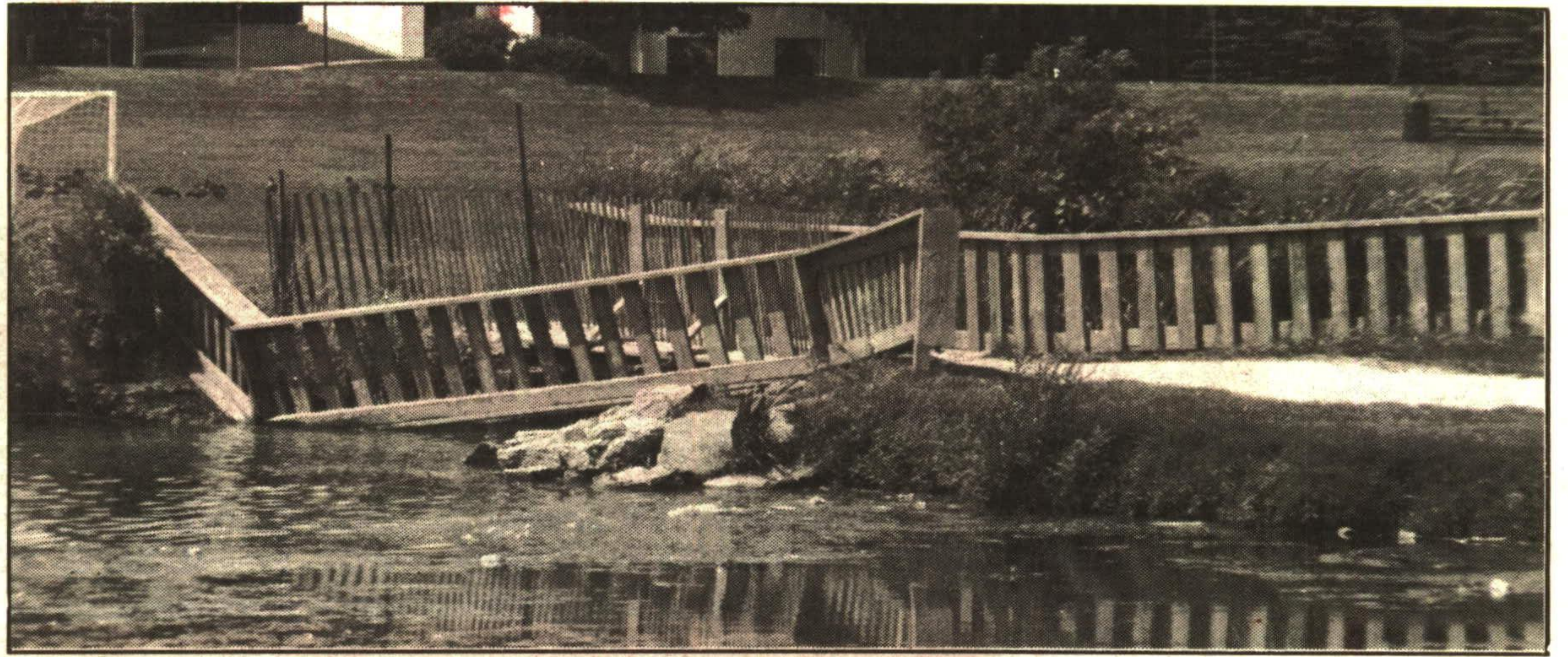
One of the railings on the bridge at Fairy Lake came off recently, and the Parks and Recreation Department has put up some temporary fencing to act as a barrier and make it safe. Parks superintendent Bryan Shynal said the
