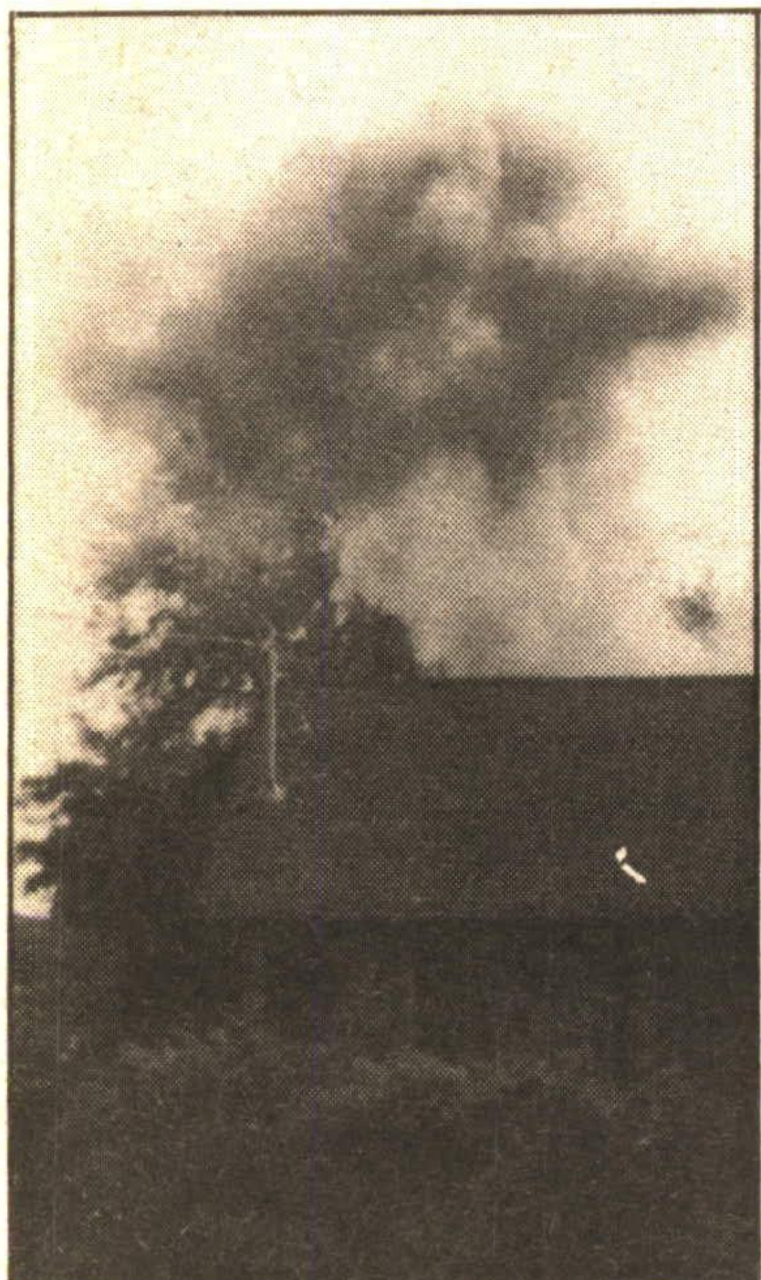
Eyewitness Mark Tait took this photo of the Mountainview Rd. hydro substation just seconds after cables exploded causing a blackout to one third of Georgetown.
