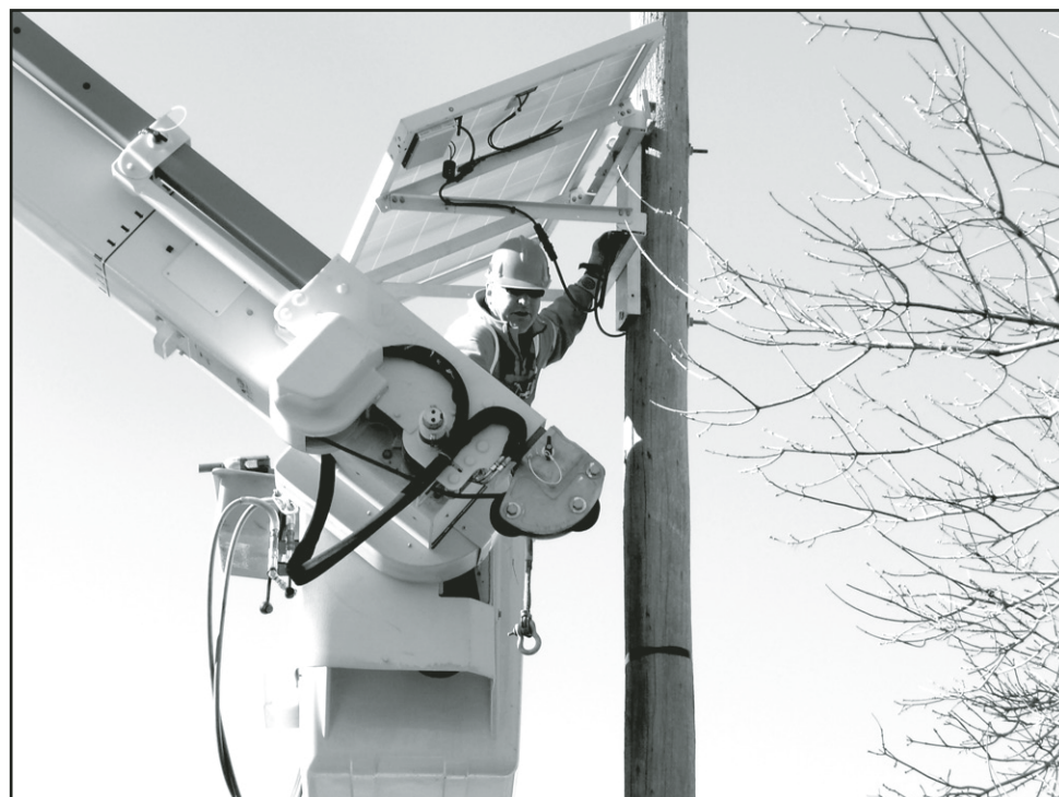
PANEL INSTALLATION: Halton Hills Hydro powerline technician Hessel Faber made installing a solar panel on a hydro pole in Ballinafad look easy last Thursday as a crowd watched at the launch of Hydro's initiative that marries renewable energy with so-called smart grid technology. - Frances Learment photo
