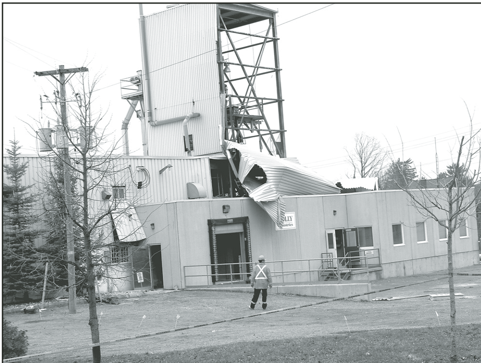
INVESTIGATION CONTINUES: The cleanup at Holly Industries on Eastern Avenue continued as investigators searched for the cause and origin of the explosion and fires at the sulphur refining plant. – Ted Tyler photo
