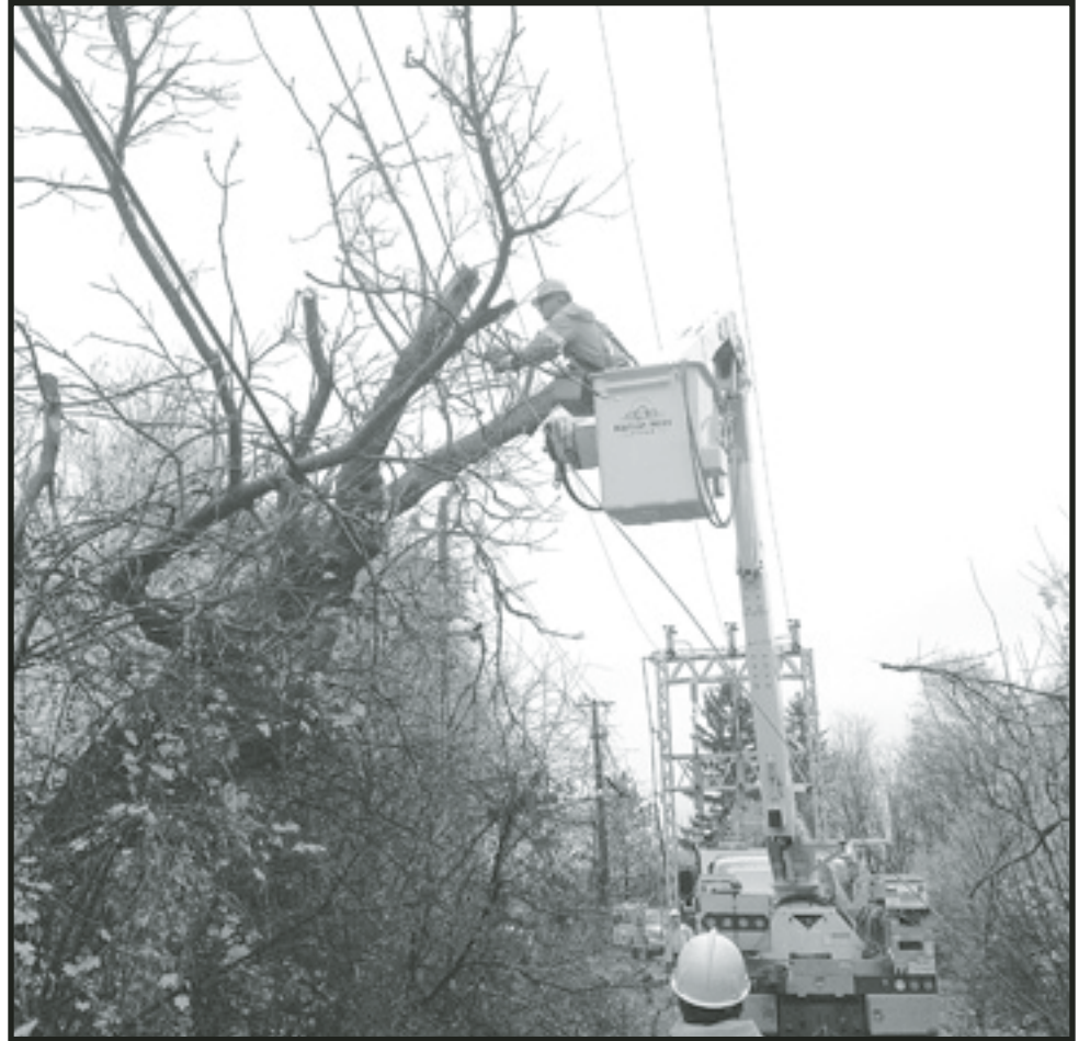
POWER OUT: Falling limbs from a rotting Manitoba Maple tree caused an hour-long power outage for 2,300 Halton Hills Hydro customers of on Monday morning in Acton. After power was isolated on the line to the Beardmore substation, crews removed the branches and made repairs. – Submitted photo
