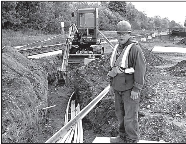
WORK PROGRESSES: Montana Electric employee Phille Bereira worked overtime recently to complete the electrical work at the under construction Acton GO Train station where service is expected in the New Year. — Frances Learment photo
