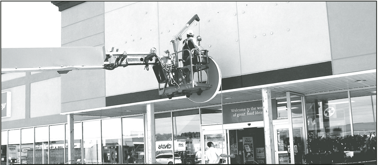
SIGN OF THE TIMES: Joe Jacques of Jones Neon Display spent most of Tuesday making sure his spelling was correct as he installed new signs at the Acton Sobeys store which is undergoing a major renovation. – Marie Shadbolt photo
