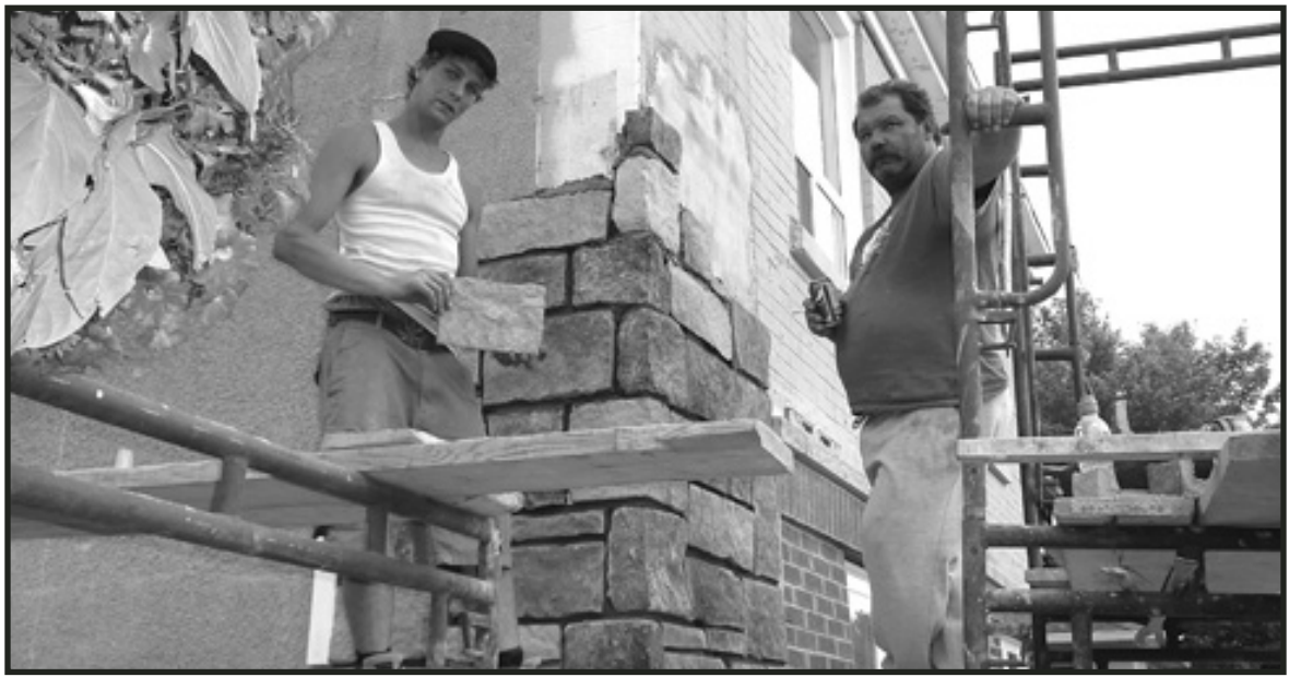
FAÇADE FIX-UP: In readiness for a new tenant – Trendz Hair Studio – at 122 Mill St. East, Mark Kri (right) owner of MK Masonry, and helper Vincent Zmija “pretty up” the front of the building. – Frances Learment photo
