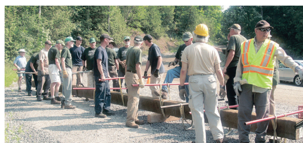
Bruce Trail enthusiasts prepare to carry in a large beam for the Silver Creek bridge.
