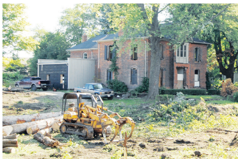
Trees around the 1870s home at 127 Mountainview Rd. N. were cut down Thursday. Photo by Ted Brown
