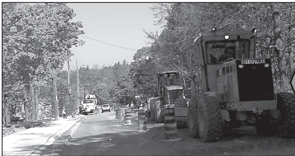
TRAFFIC WOES: Construction season has Hwy. 7 through Rockwood torn up causing delays for traffic in both directions. - Marie Shadbolt photo
