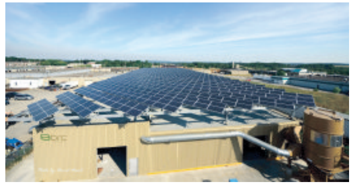
An overhead view shows the newly installed solar panels on the BRC Business Enterprises 35,000 square-foot manufacturing facility on Armstrong Ave. in Georgetown. The panels are expected to generate enough electricity to power 30 homes for a year.
