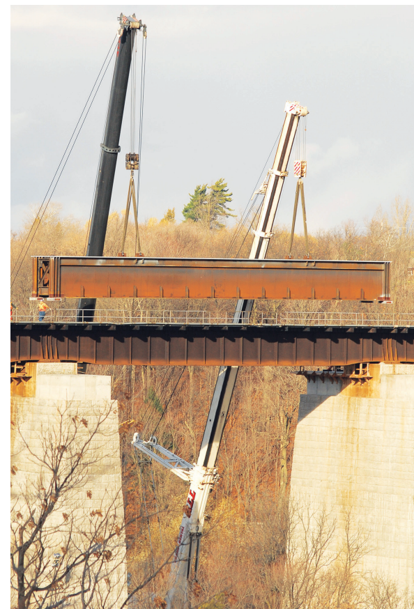
CN Rail crews were busy installing a segment of bridge on the trestle over the Credit River in Georgetown last week.
