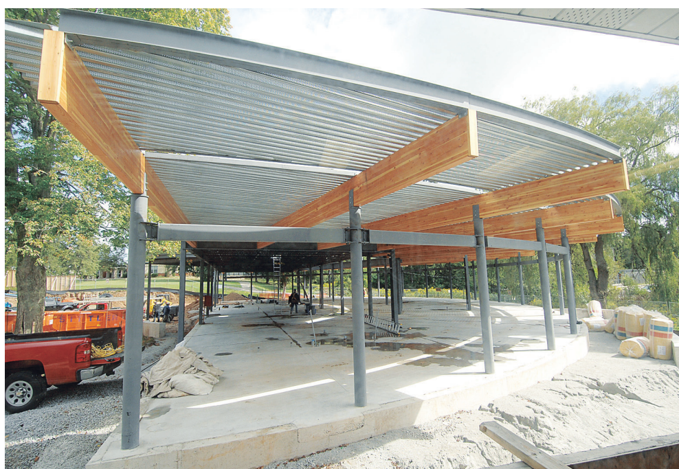
Work is progressing nicely on the new Acton branch of the Halton Hills Public Library with the wood roof beams now installed. Photo by Ted Brown
