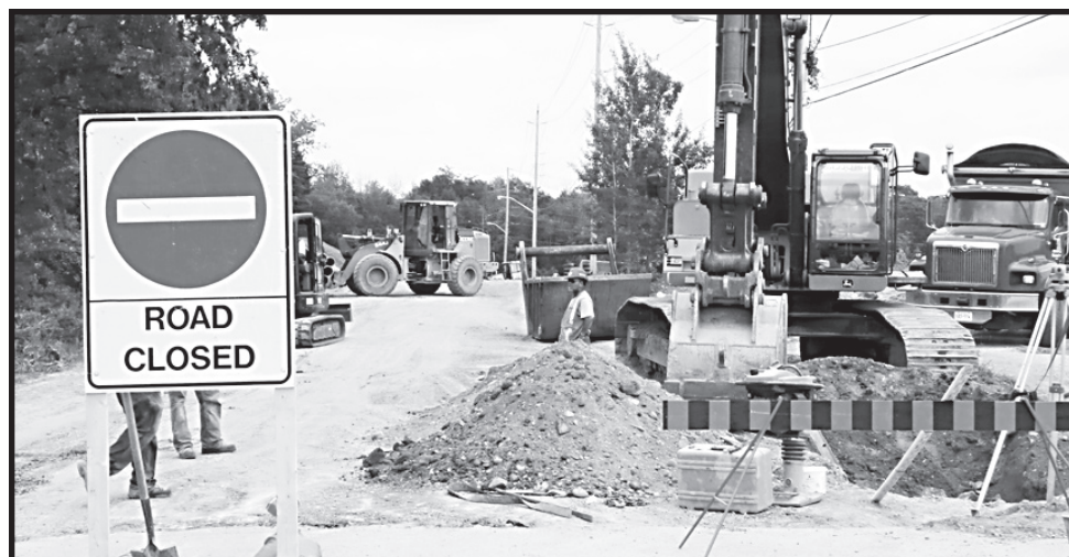
TRAFFIC HEADACHES: It will be a long summer of traffic hassles for motorists in Acton who must deal with the reconstruction closure of Wallace Street, from Dr. Moore Crescent to McDonald Boulevard, and with watermain replacement on Queen Street from Eastern Avenue to Churchill Road. – Frances Niblock photo
