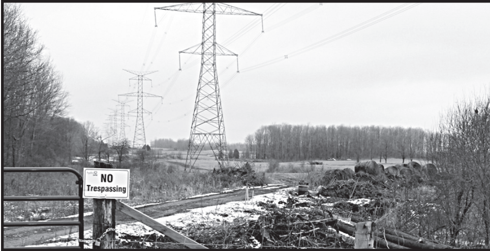
PREP WORK: Hydro One crews are building access roads in the Acton area, preparing for construction of the twinned power line from Bruce to Milton. – Frances Niblock photo
